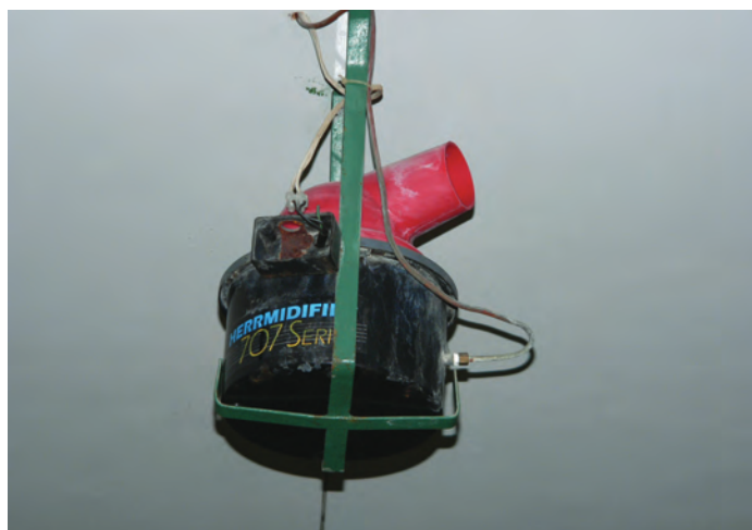
A storage room humidification unit
